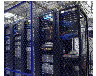
Fig 1. Snapshot of Row of a Typical Data Center
